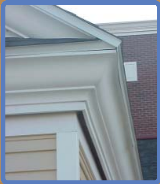
Crown and frieze board built out and with screen installed to provide ventilation
