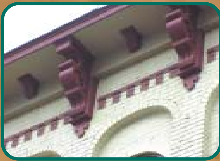
These large brackets were supplied as part of the historic restoration project on the Peck Building in Grand Rapids, Michigan.
